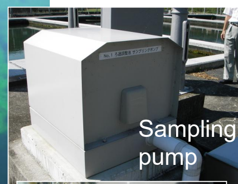
Good filter condition
