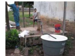
Pump for groundwater and source water tank
