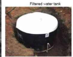
Filtered water tank
