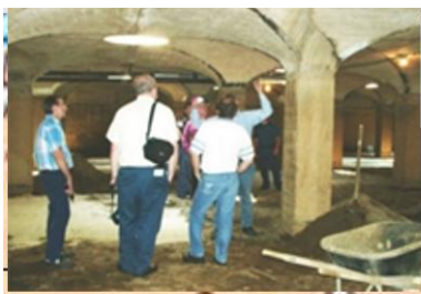
Covered filter, Albany, NY, US
