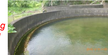
Up-flow Roughing Filter:
